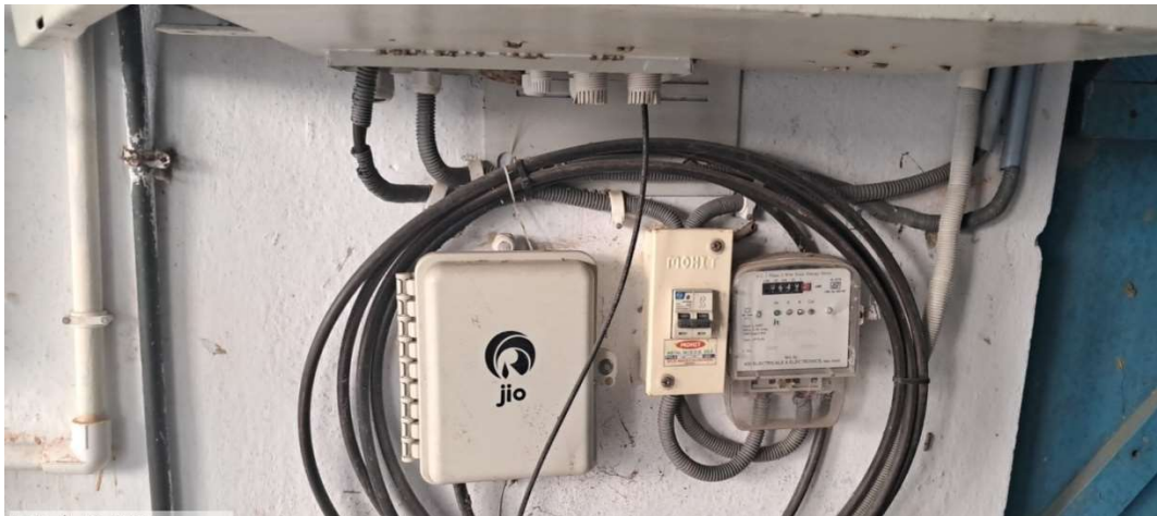
Insulated electric meter at Ramnagar College
