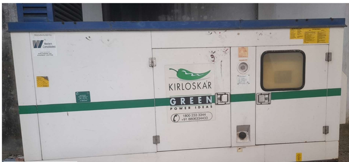
Emergency supply line at Ramnagar College
